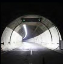
ARCALED SERIES MASSINO VISCONTI TUNNEL Novara - Italy
